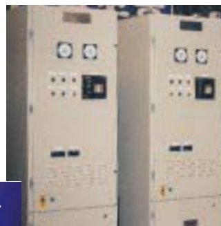
Two of the 486 3.3kV Starter Panels manufactured by Hyundai incorporating P&B Relays for the Great Man-Made River Project in Libya.
